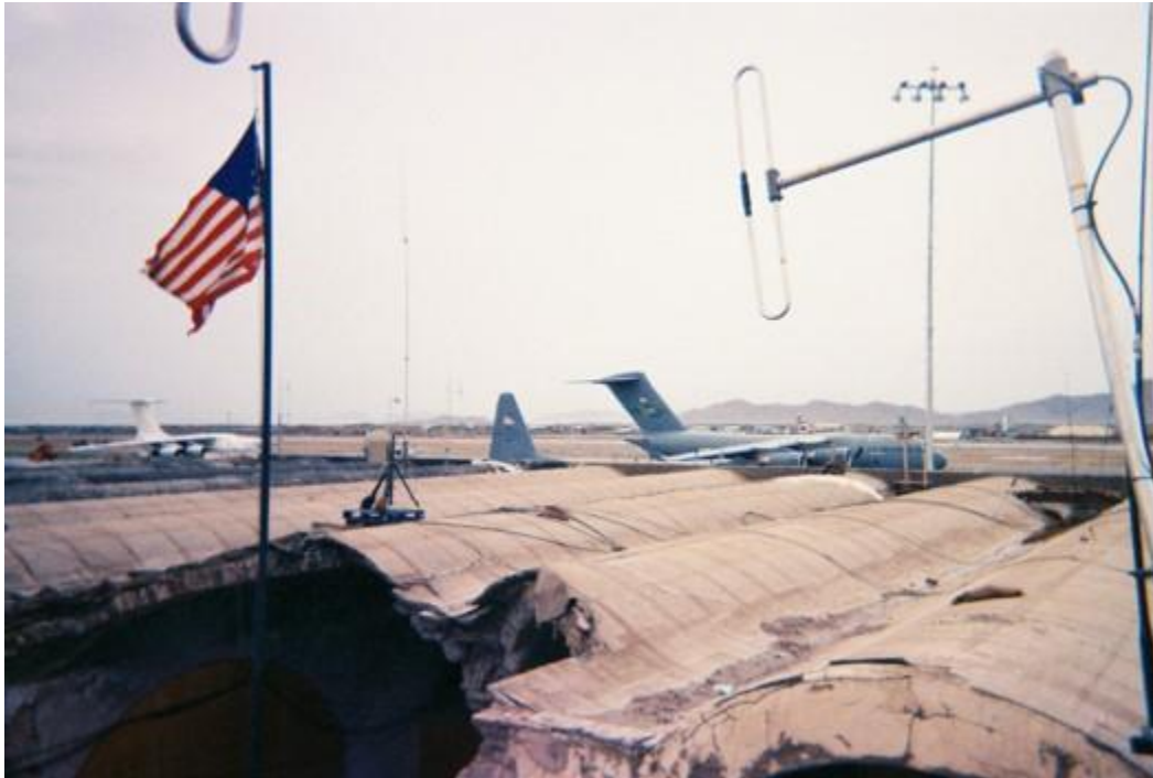
The TLS roof observation deck (bomb damage), with Russian and American aircraft © Stephen Meloche
